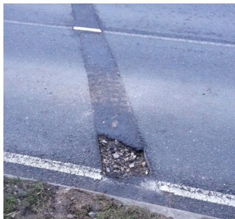
An example of poor & unfinished reinstatement work along a duct trench near Mentmore in 2015.
